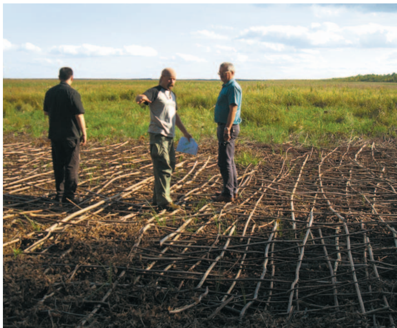
▲ Fig. 4.4.12 Crosswise arranged fascines from bushes can stabilise frequently used tracks, Biebrza Valley, Poland, September 2009 (photo: L. Lachmann).
