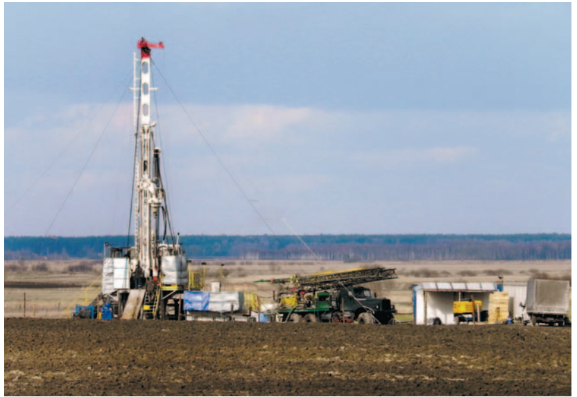
▲ Fig. 3.19 Exploratory drilling for coal close to the Bubnów Marsh, Poland, February 2016 (photo: G. Grzywaczewski).
